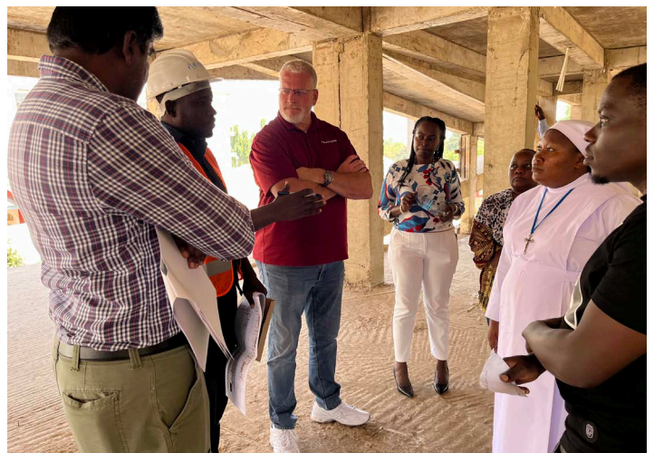
Ratish Kumar (biomedical engineer) and Darin Gardner (center) tour the structure of the new St. Joseph mother/baby building with the architect and St. Joseph administrators.
